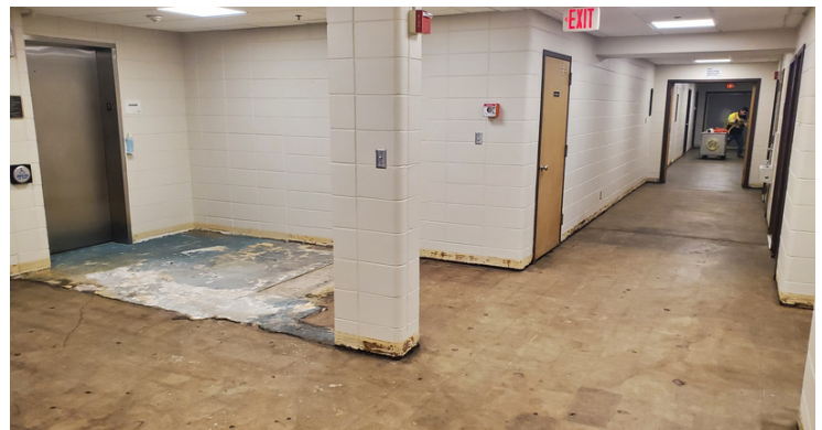
The carpet in the downstairs hallway was removed along with all of the asbestos tile. (Dec. 26, 2023) Ready to start 2024 with fresh, smooth carpet!
